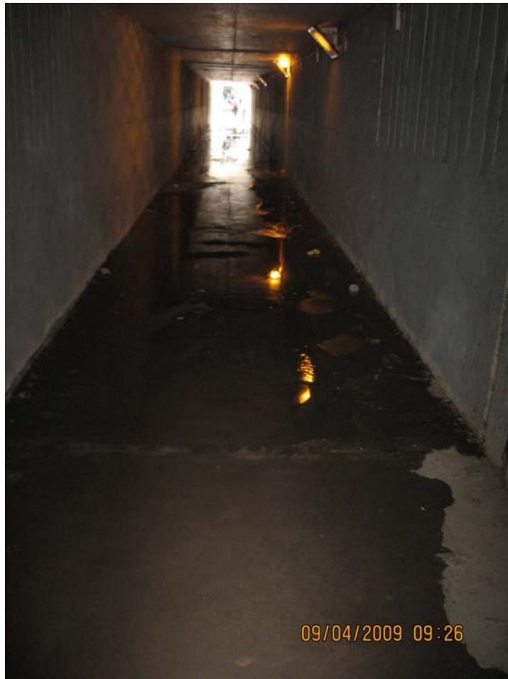
Pedestrian Underpass Ponding
