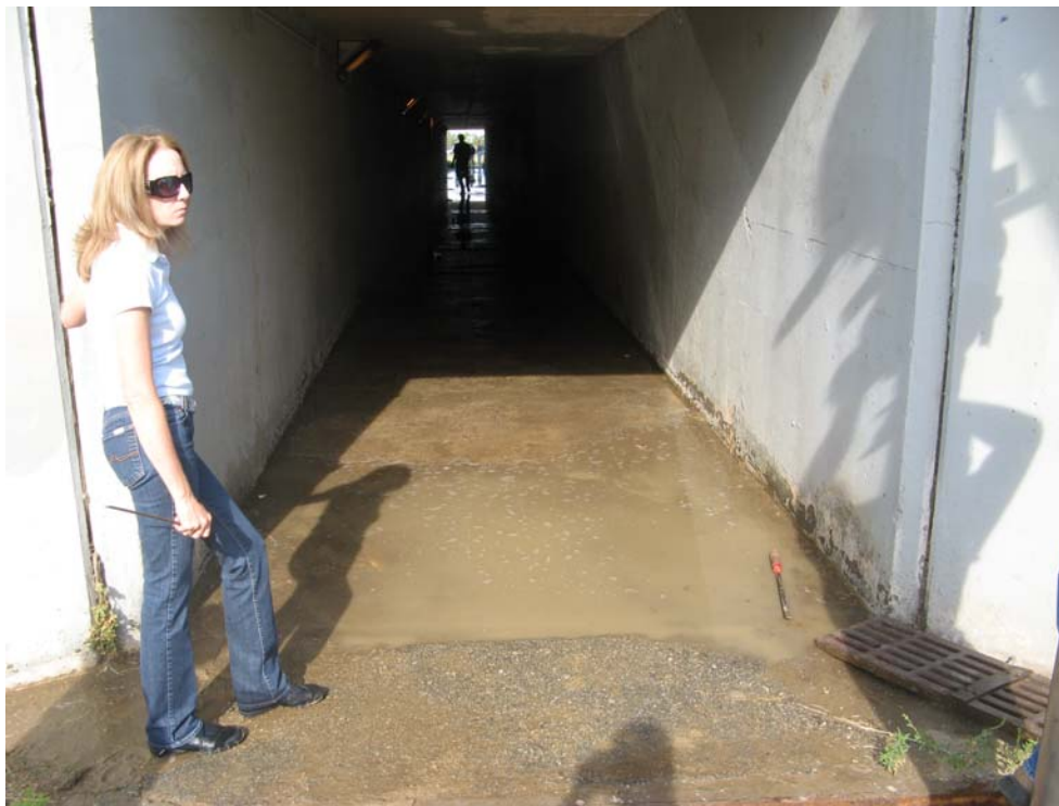
Pedestrian Underpass - East End Ponding
