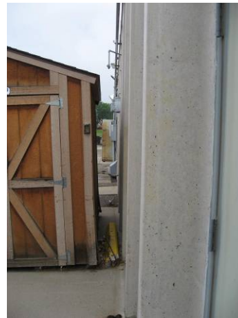
Inadequate Building Separation
