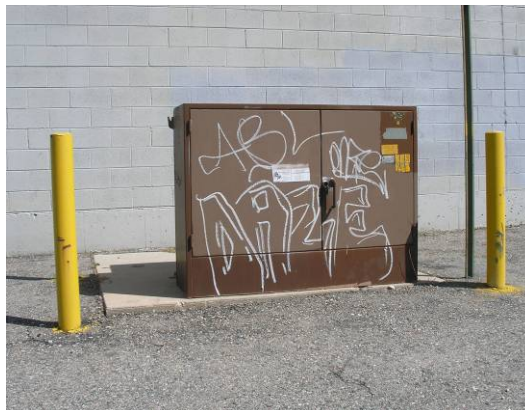
Graffiti on Utility Box
