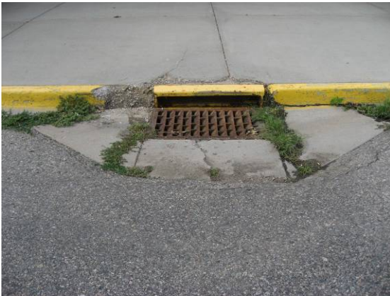
Broken Curb & Gutter
