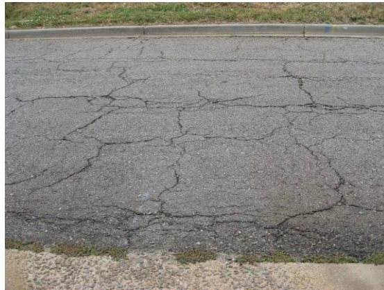
"Alligator" Cracking in Parking Lot
