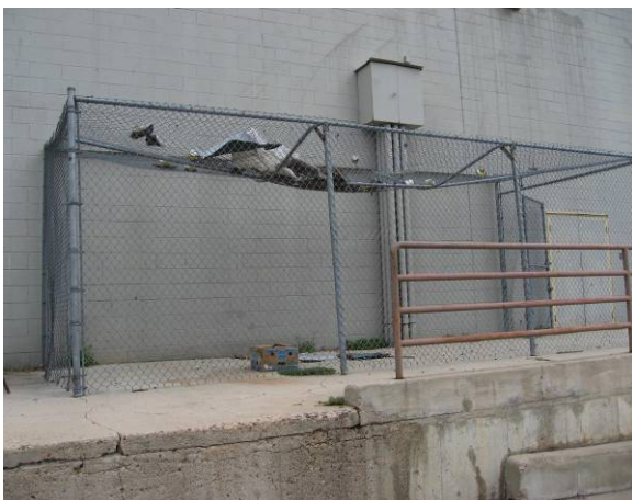
Trash & Debris Atop Fence Enclosure
