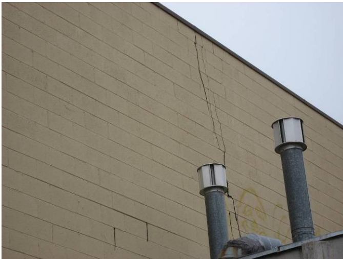
Cracked Wall of Anchor Building
