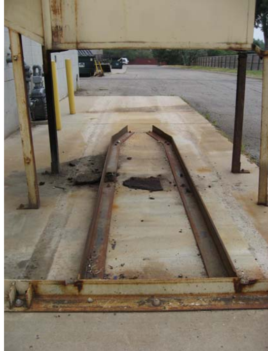
Broken & Rusting Trash Chute
