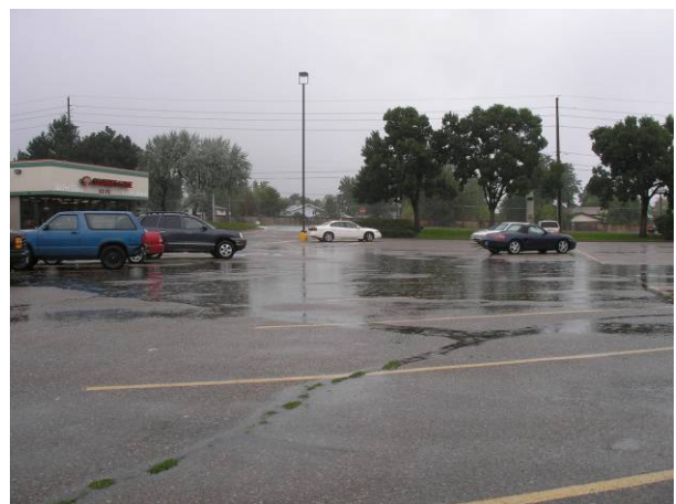
Standing Water in Main Parking Lot
