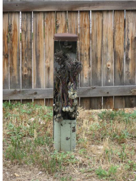
Exposed & Stripped Utility Box
