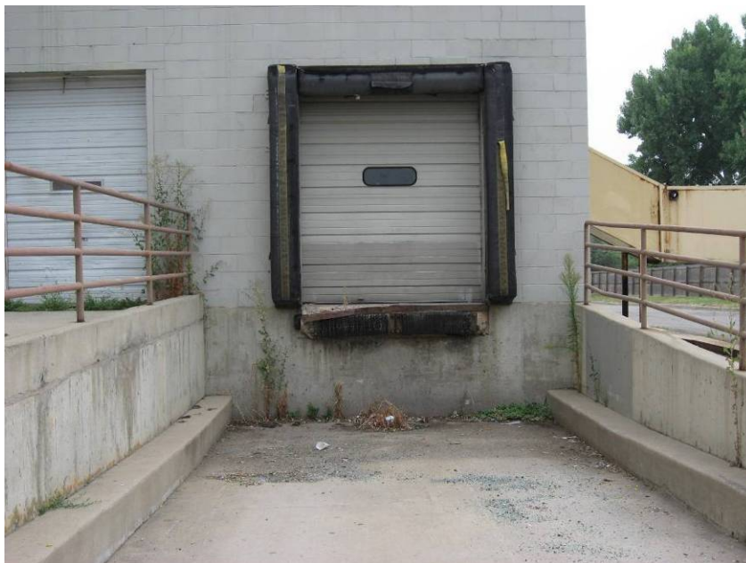
Deteriorating Loading Dock
