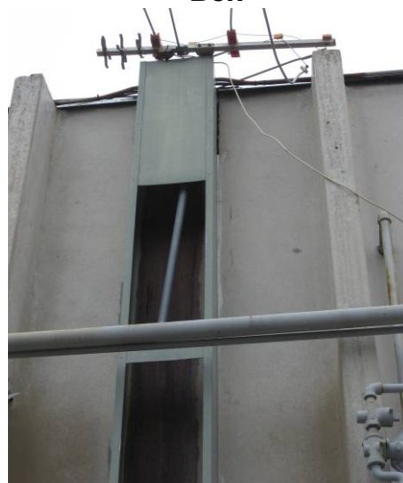
Cable Antennae Improperly Installed & Secured
