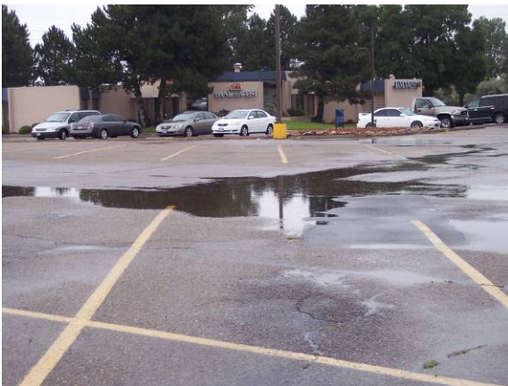
Standing Water in Main Parking Lot
