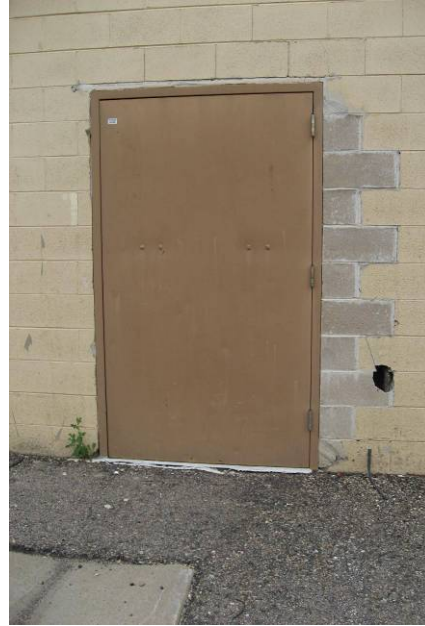
Door Lacking Hardware
