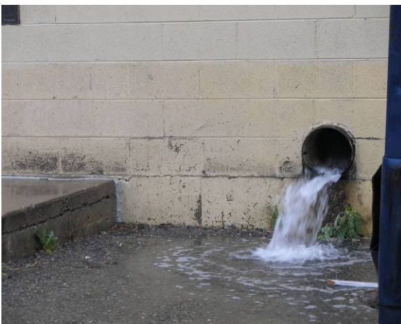
Roof Drain Emptying at Base of Building
