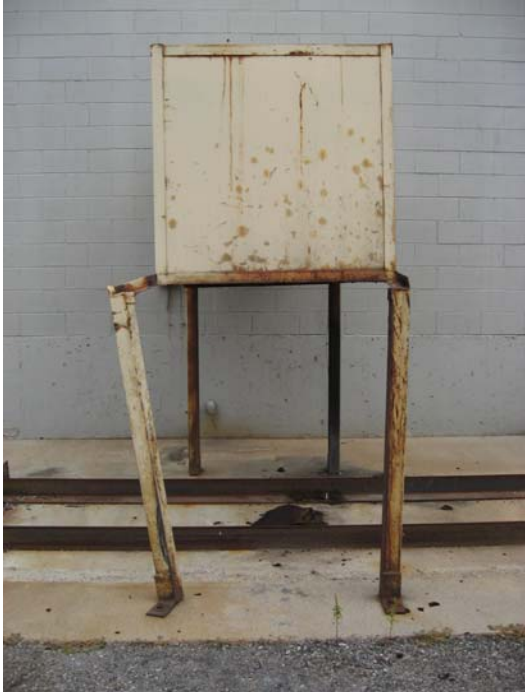
Broken & Rusting Trash Chute
