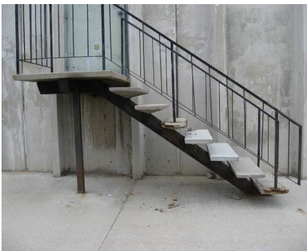
Broken & Rusting Stairs
