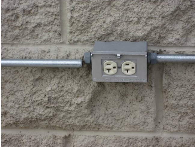
Exposed Electrical Box & Wiring
