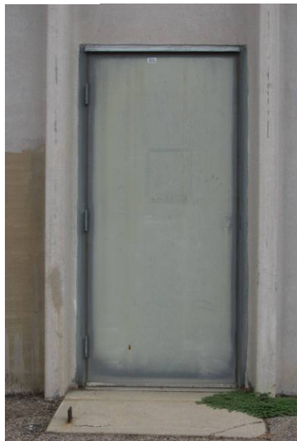
Door Welded Closed
