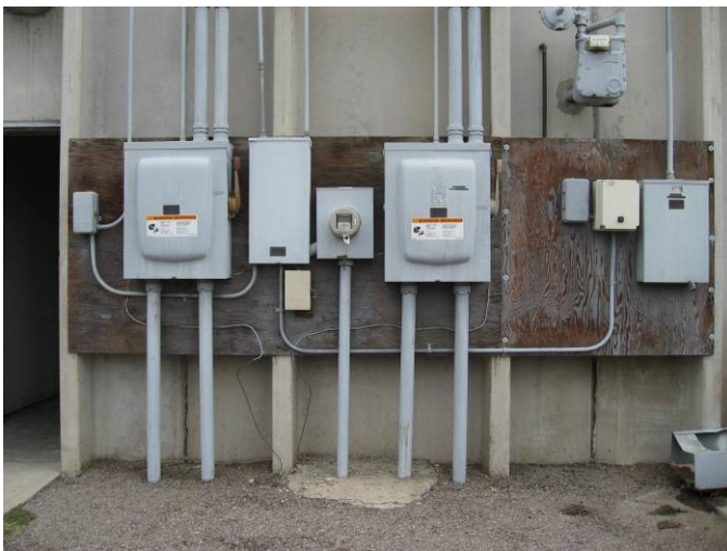
Electrical System Improperly Mounted to Rotting Plywood
