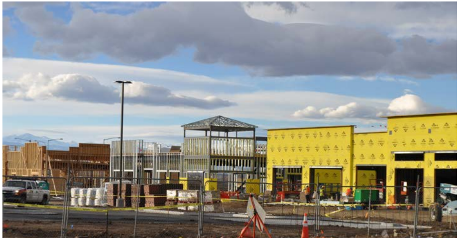
Construction of seven buildings at Webster Lake Promenade. Nine new restaurants and other retail and service businesses are scheduled to open in mid to late 2014.
