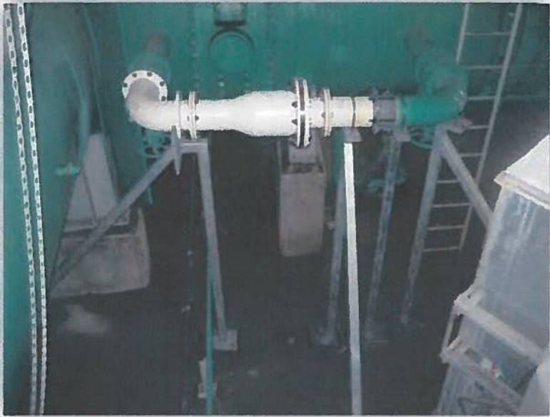
New By-pass line in Standley Lake Valve House
