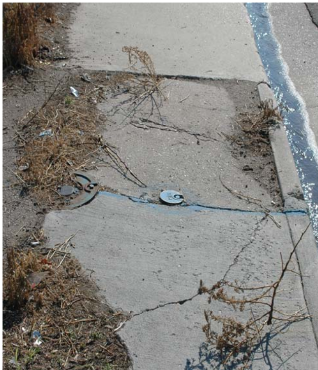
5.6.2. Water meter located in sidewalk.
