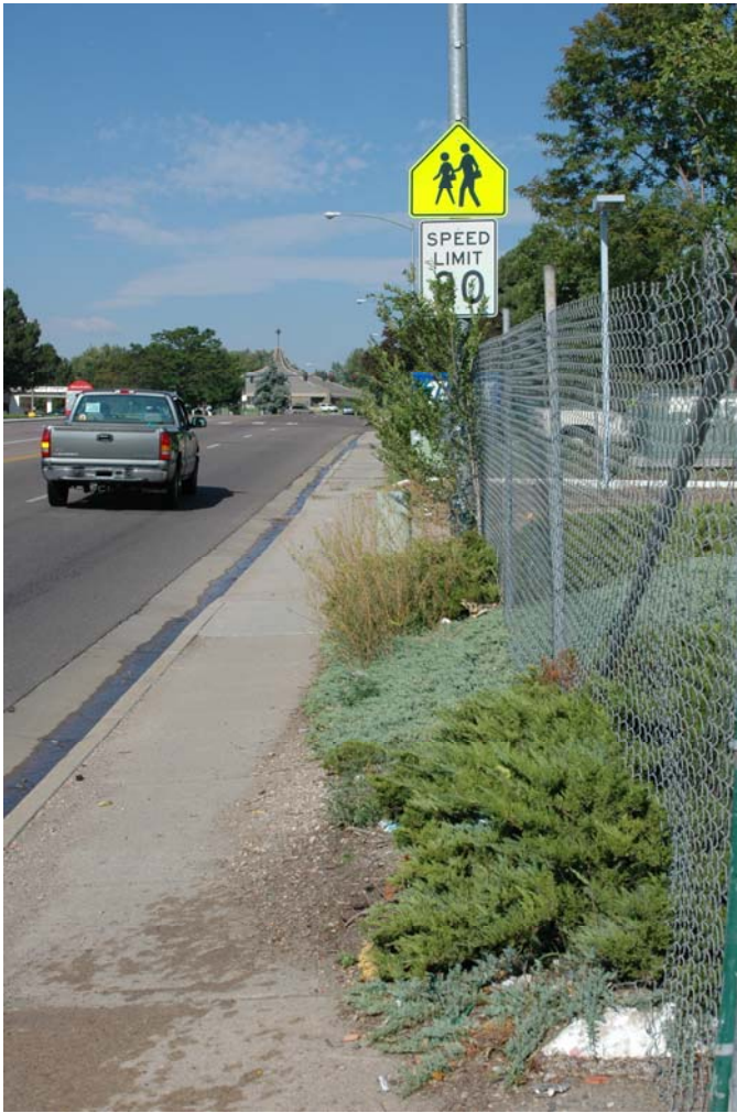
5.4.7. Eroded soil and gravel on sidewalk.
