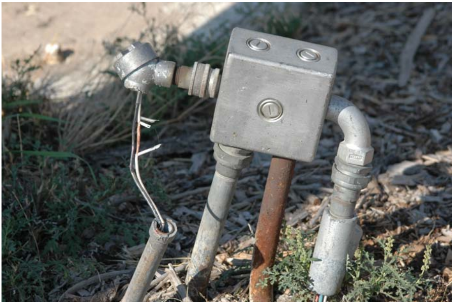
5.4.8. Exposed electrical wiring.
