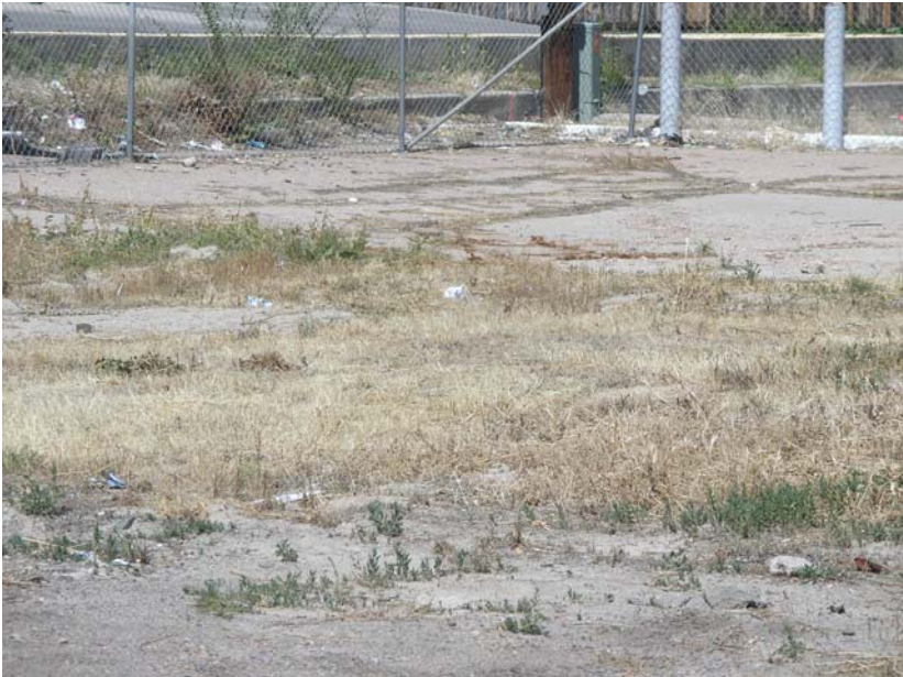
5.5.2. General site deterioration.
