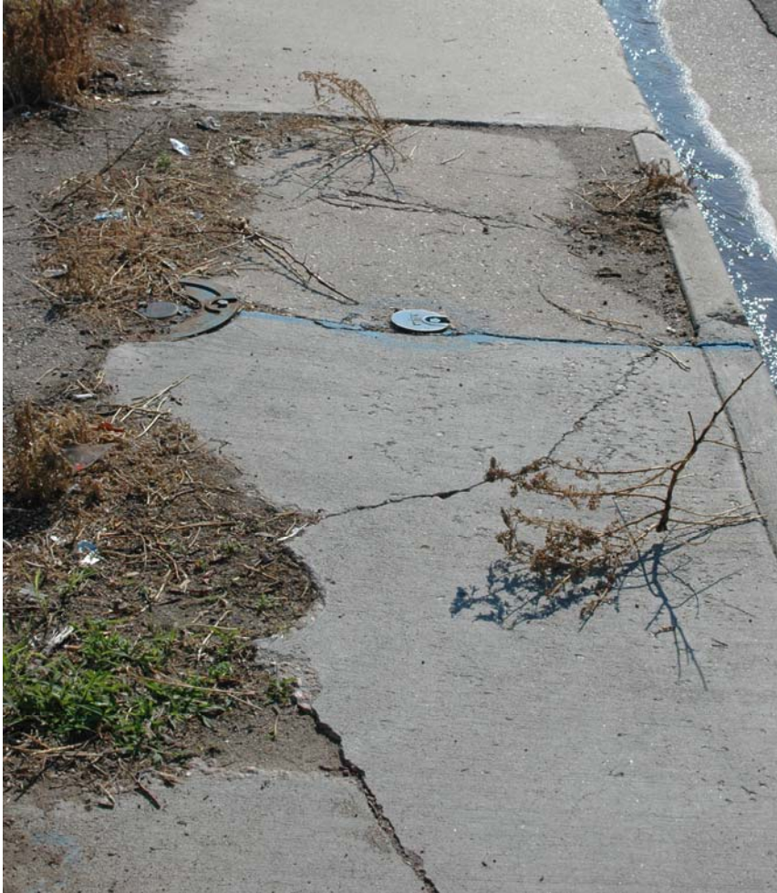
5.4.1. Broken sidewalk adjacent to site.
