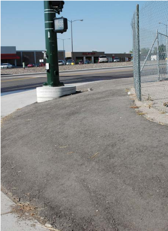
5.6.1. Excessive slope adjacent to public street.
