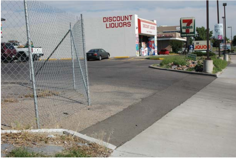
5.4.3. Fence obstructing shared driveway.
