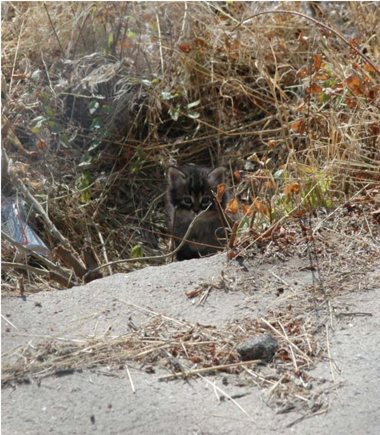
5.4.5. Broken concrete drive and cavities underneath Sheltering stray and feral animals.
