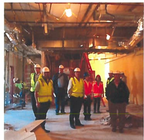
IECRM team begins major remodel and renovations of new facility at 11429 Pearl St.
