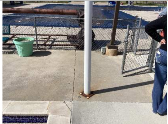
Photo #6: 120V Light pole base installed near shallow pool. Verify conduits to and from light pole base meet distance requirements from water's edge.
