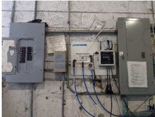
Photo #1: Panel HPA & LPA
