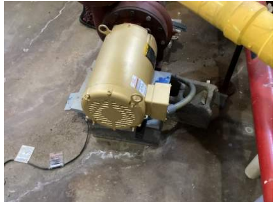
Photo #2: Grounding conductor not found to be attached at pump motor
