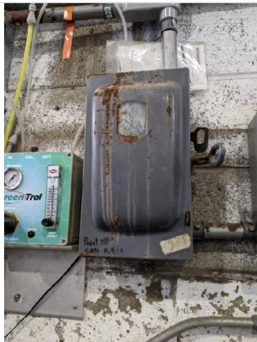
Photo #4: Rust damage on electrical disconnect
