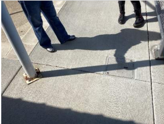
Photo #5: Electrical junction box found near shallow pool and shade structure.
