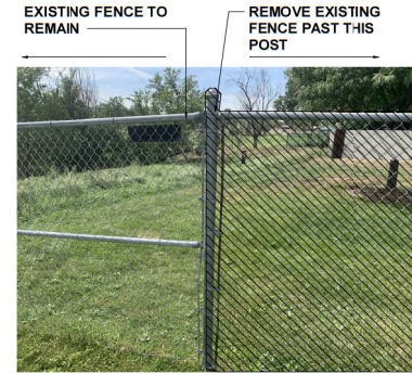
21 EXISTING FENCE DETAIL VIEW T-100
