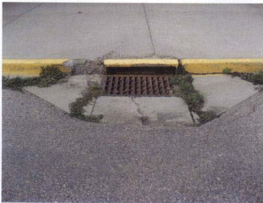
Broken Curb & Gutter
