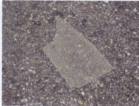
Broken Glass in Parking Lot
