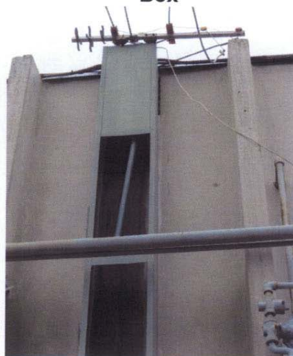
Cable Antennae Improperly Installed & Secured
