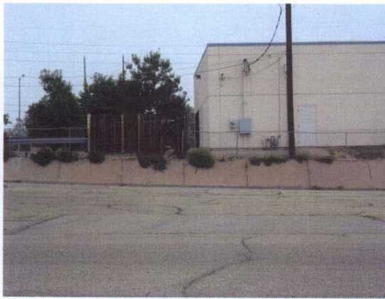
Slope of Parking Lot
