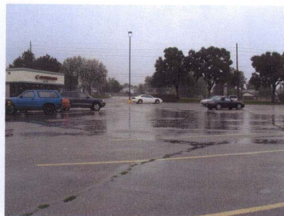
Standing Water in Main Parking Lot
