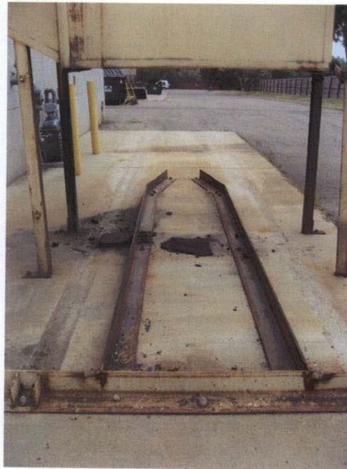
Broken & Rusting Trash Chute
