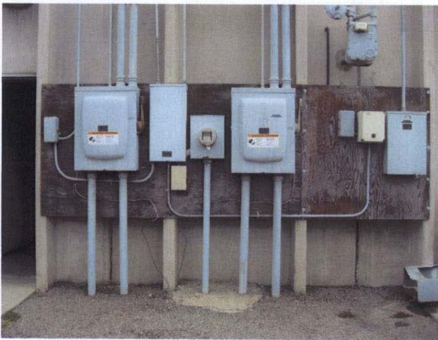
Electrical System Improperly Mounted to Rotting Plywood
