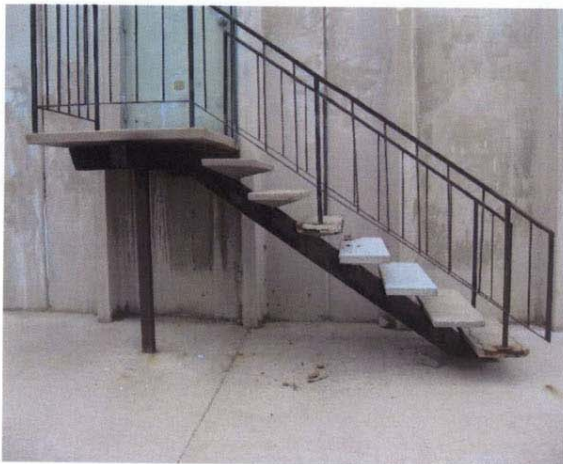
Broken & Rusting Stairs
