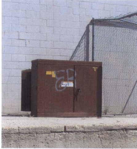
Graffiti on Utility Box
