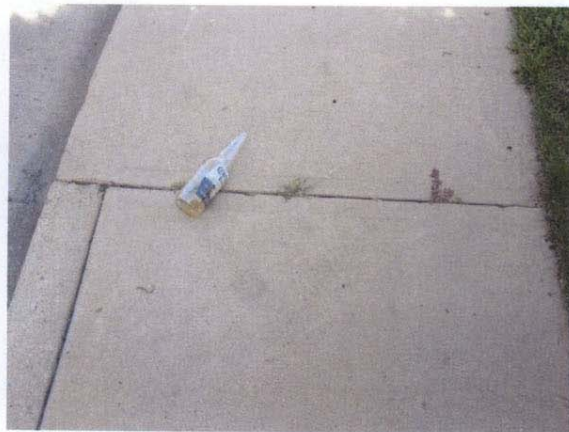
Trash Along Sidewalk
