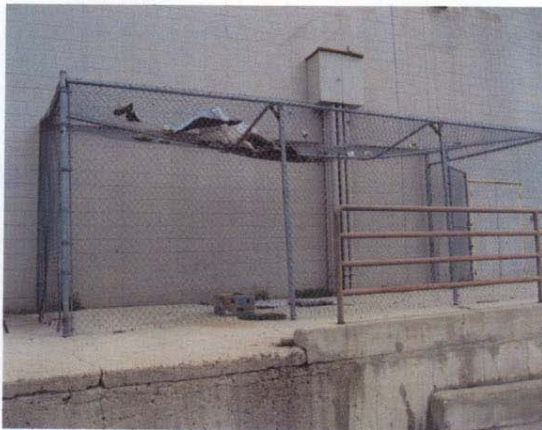
Trash & Debris Atop Fence Enclosure
