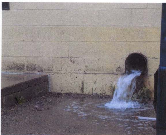
Roof Drain Emptying at Base of Building
