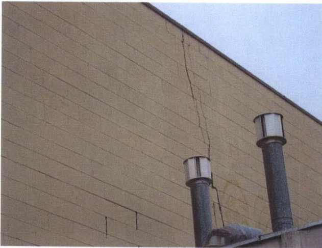
Cracked Wall of Anchor Building
