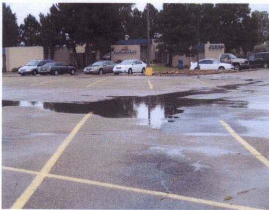
Standing Water in Main Parking Lot
