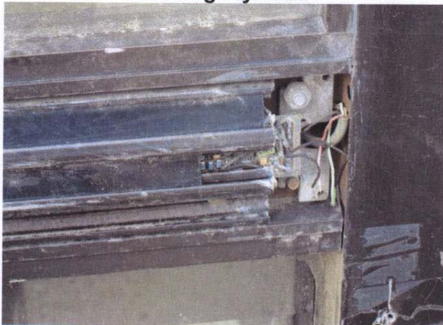
Exposed Electrical Wiring
