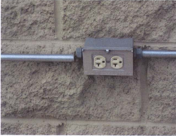
Exposed Electrical Box & Wiring
