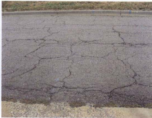
"Alligator" Cracking in Parking Lot
