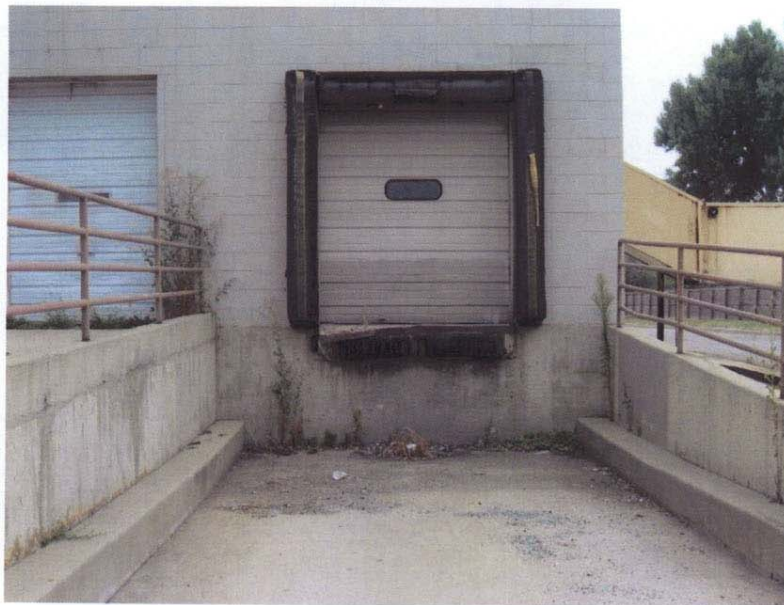
Deteriorating Loading Dock
