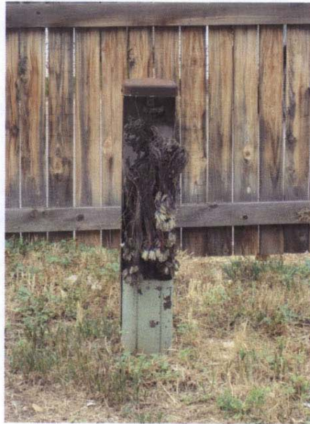
Exposed & Stripped Utility Box
