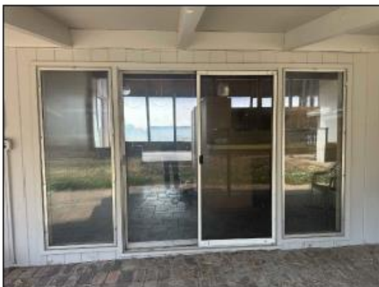
Sliding Glass door is not original the 2 side windows are but not tempered glass
