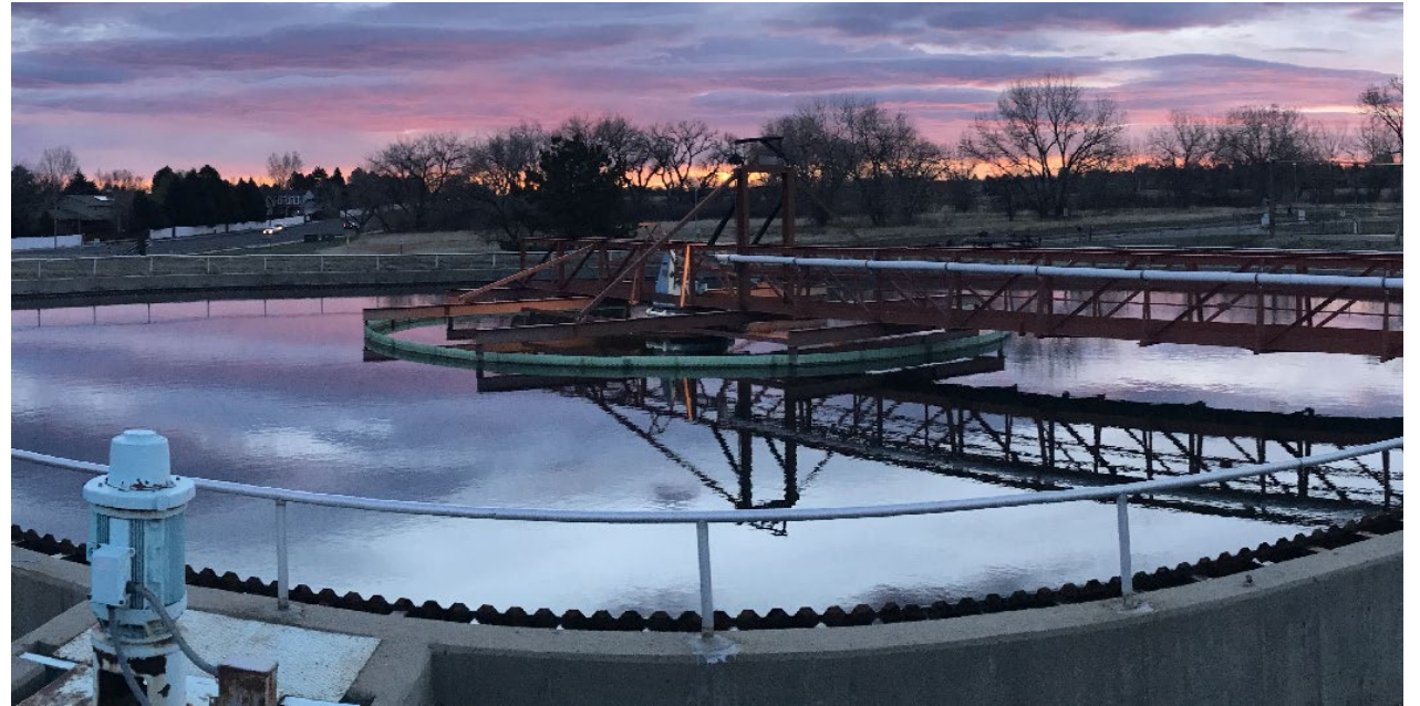
Water Treatment Facility
