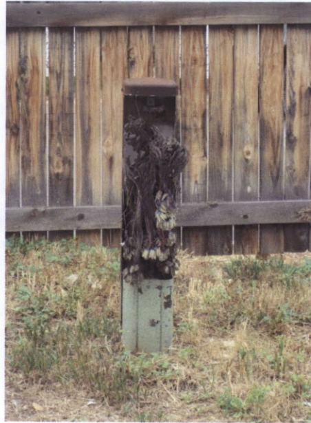
Exposed & Stripped Utility Box
