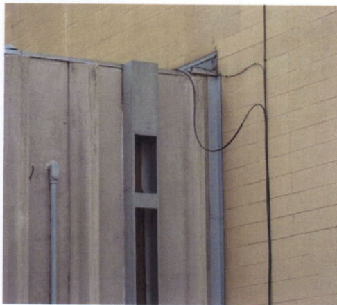
Exposed Live Wire
