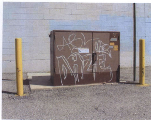
Graffiti on Utility Box
