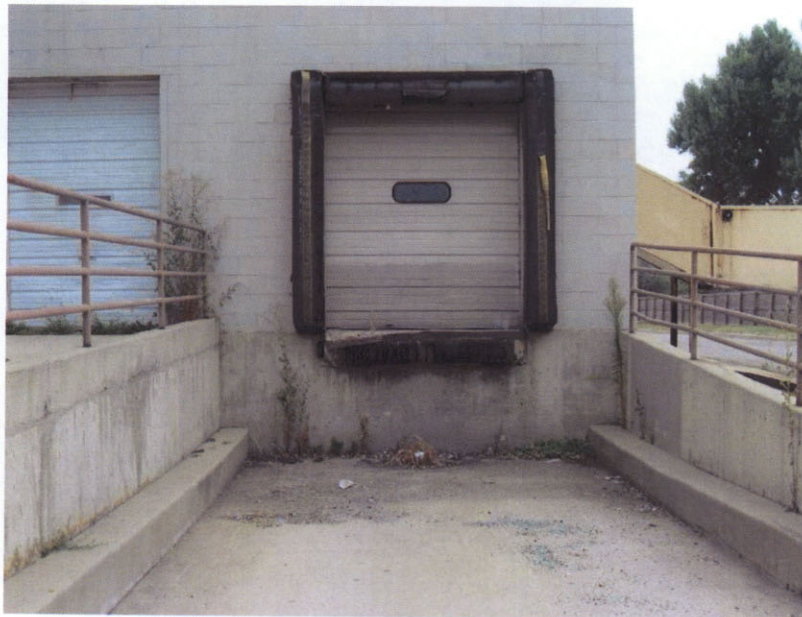
Deteriorating Loading Dock
