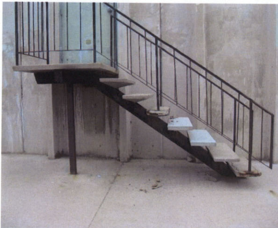
Broken & Rusting Stairs
