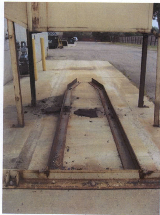
Broken & Rusting Trash Chute
