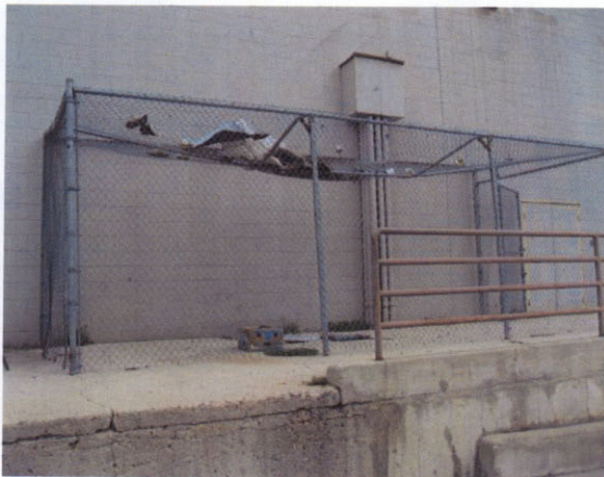
Trash & Debris Atop Fence Enclosure
