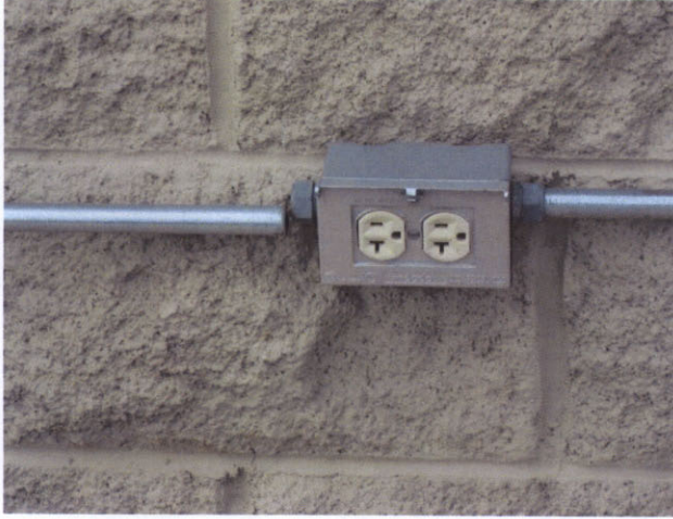
Exposed Electrical Box & Wiring
