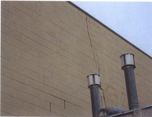
Cracked Wall of Anchor Building
