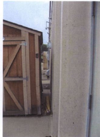
Inadequate Building Separation
