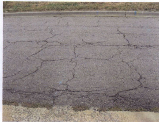
"Alligator" Cracking in Parking Lot
