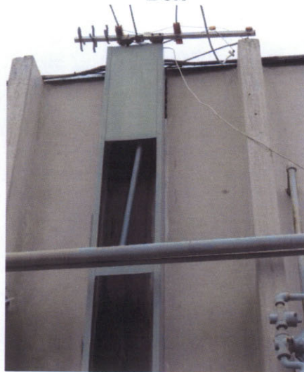
Cable Antennae Improperly Installed & Secured
