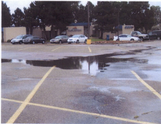
Standing Water in Main Parking Lot
