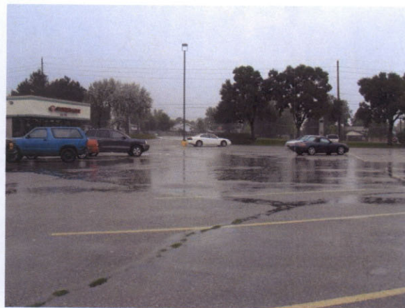
Standing Water in Main Parking Lot
