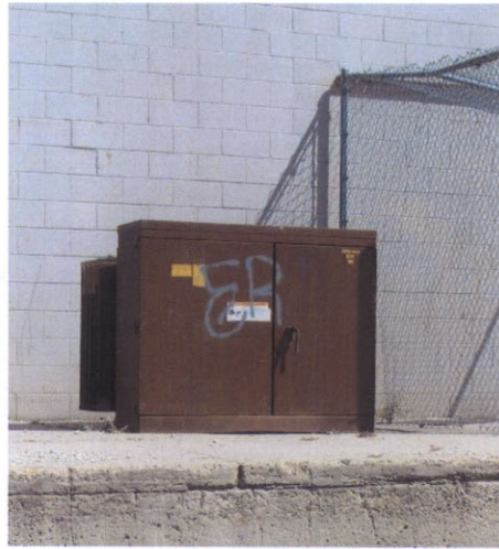
Graffiti on Utility Box
