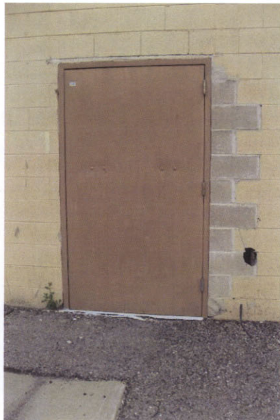
Door Lacking Hardware
