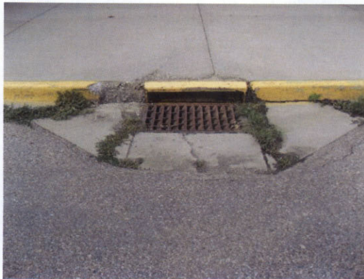
Broken Curb & Gutter
