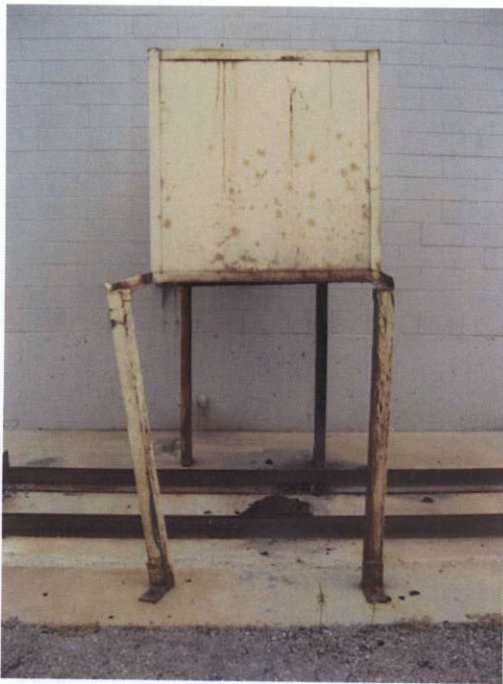
Broken & Rusting Trash Chute
